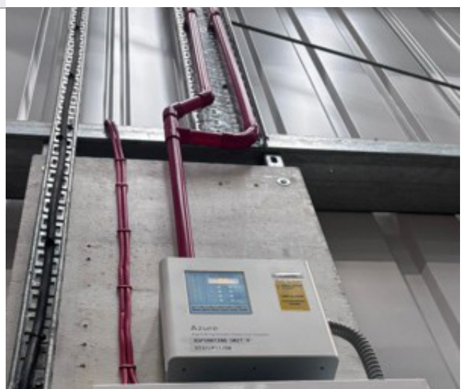
Sensis Azure 2000s Control Panel connected to sampling pipe network in distribution centre [courtesy of Procester Fire & Security]
