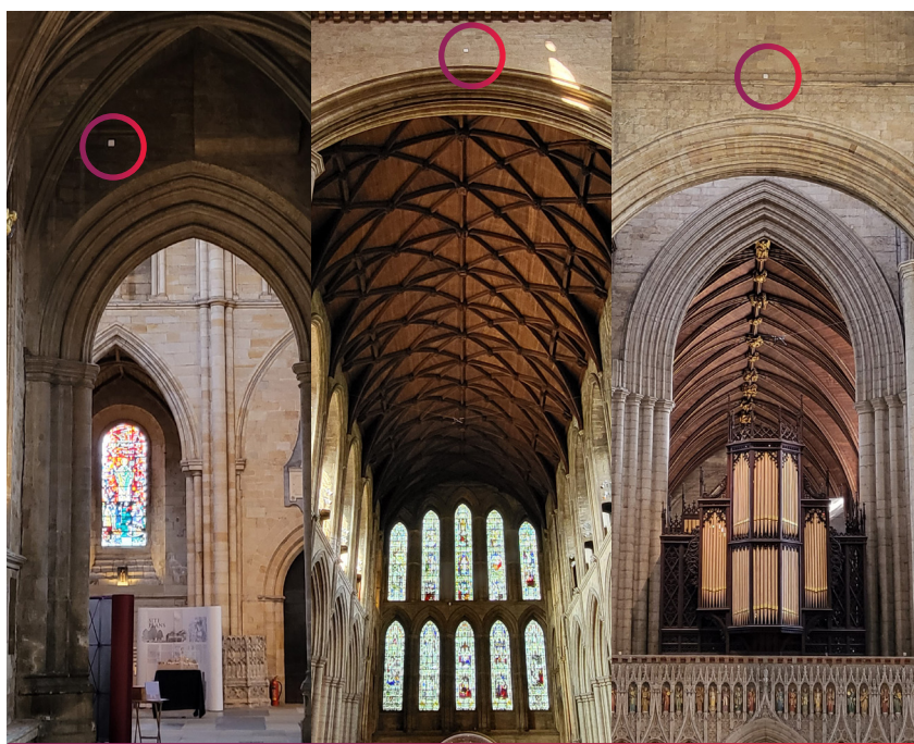
Reflector positions in the cathedral (Images courtesy of Charles Thomas Heritage Fire Protection Specialists Ltd)
